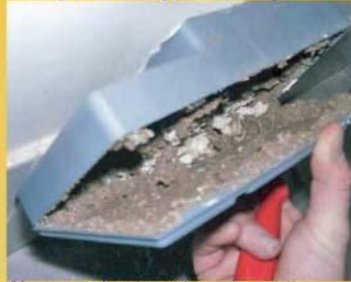
Above ground station with termite activity.
