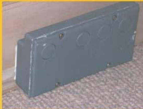
Above ground station placed on damaged wall.
